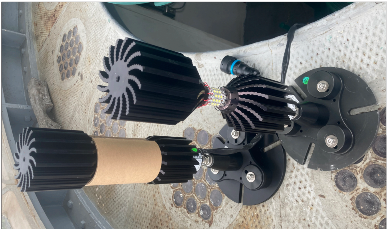
Oct., 2022 - replacement LED light with older lightning struck LED (Ralph Krugler)
