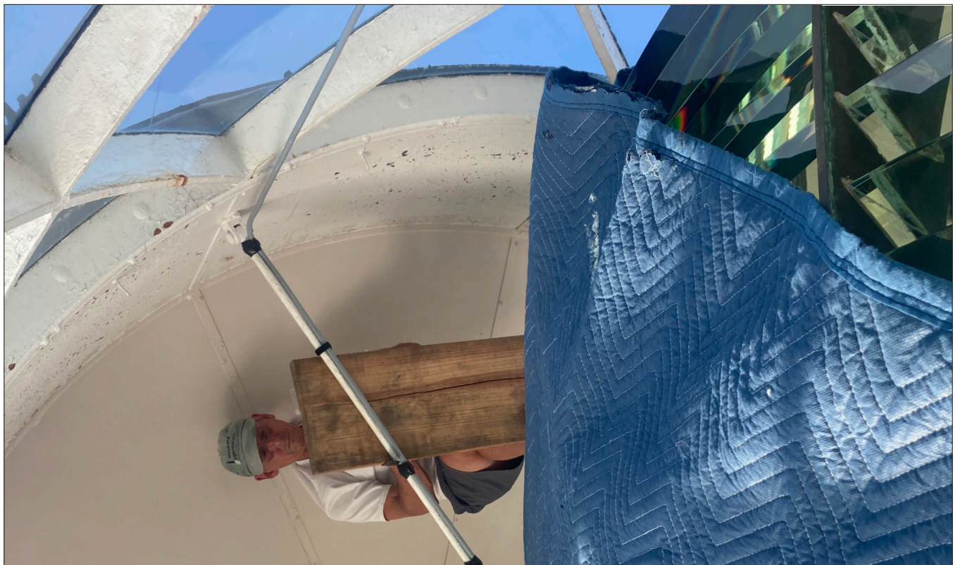
May 21, 2021 - Ken Herman installing the new LED power cable over the lens (Ralph Krugler)
