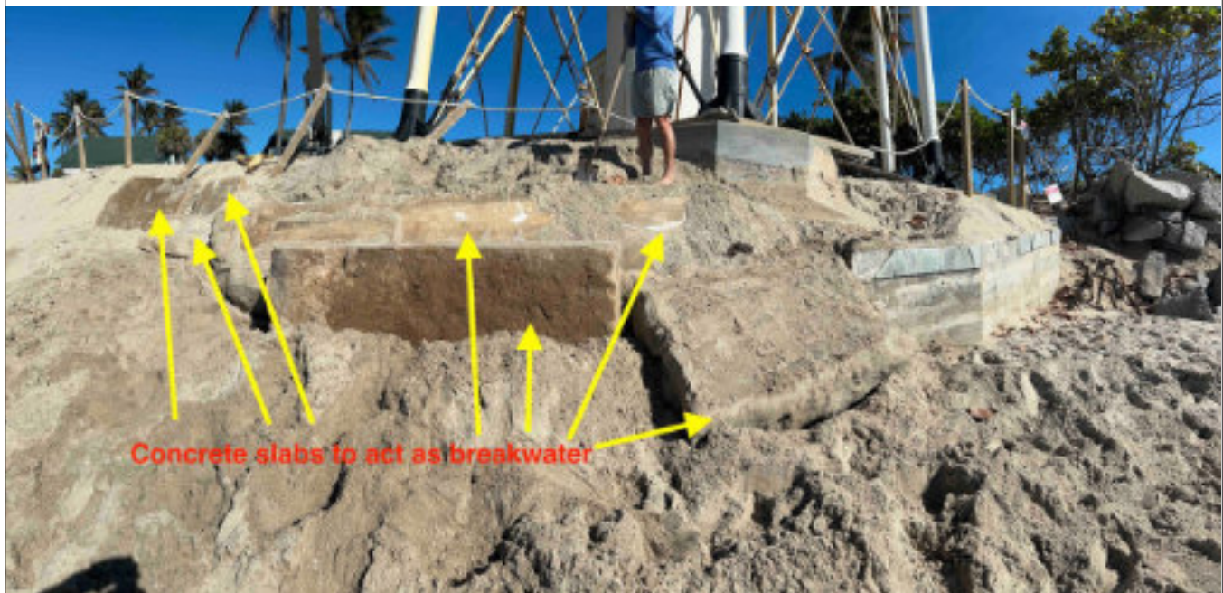
October, 2024 - Erosion at the Lighthouse (Ralph Krugler)
